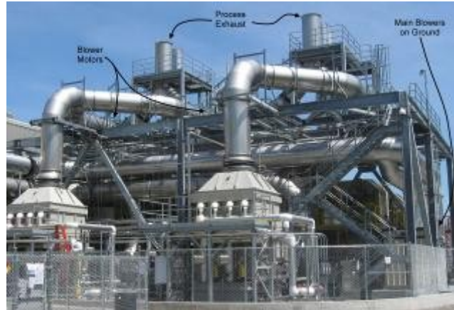
Thermal Oxidizers in rear utility yard.
