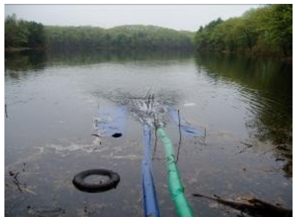
Pump test groundwater discharge to Mirror Lake
